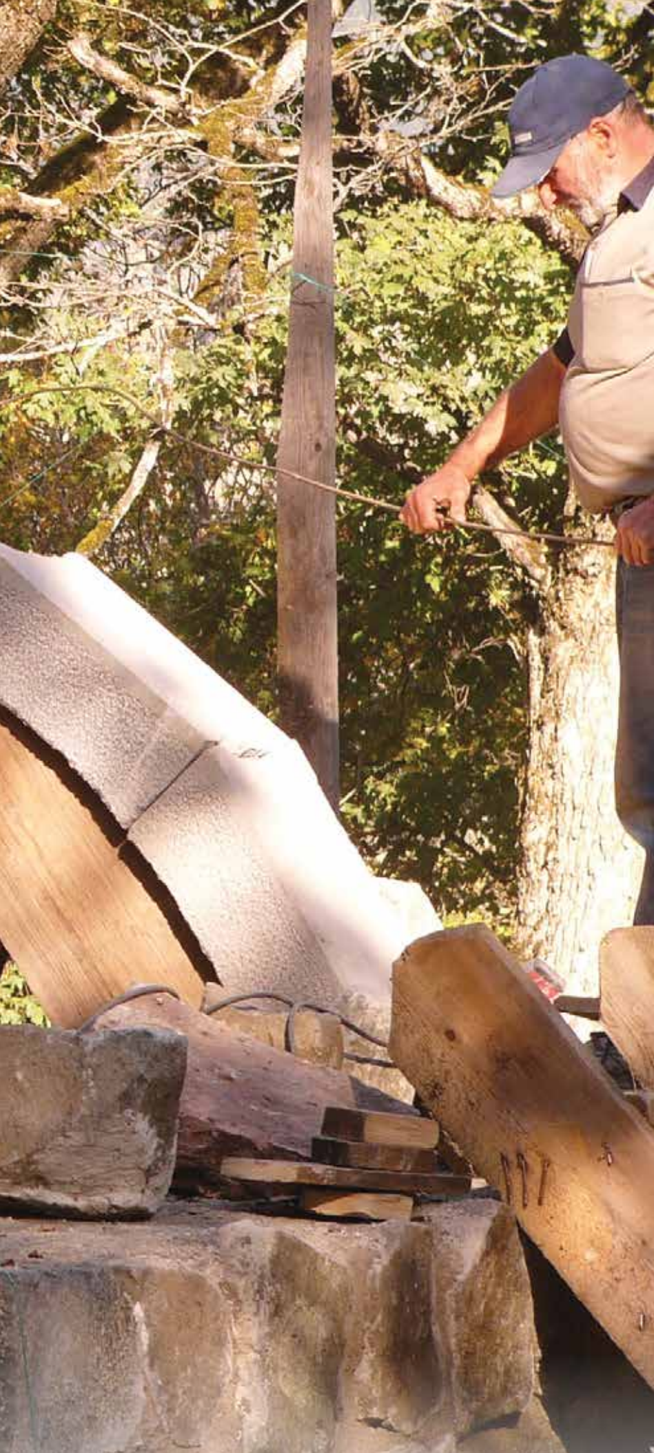
Restoring the domed roof of St. Mary's Church at Tadzrisi in Georgia involved replacing missing stones and securing loose ones.
