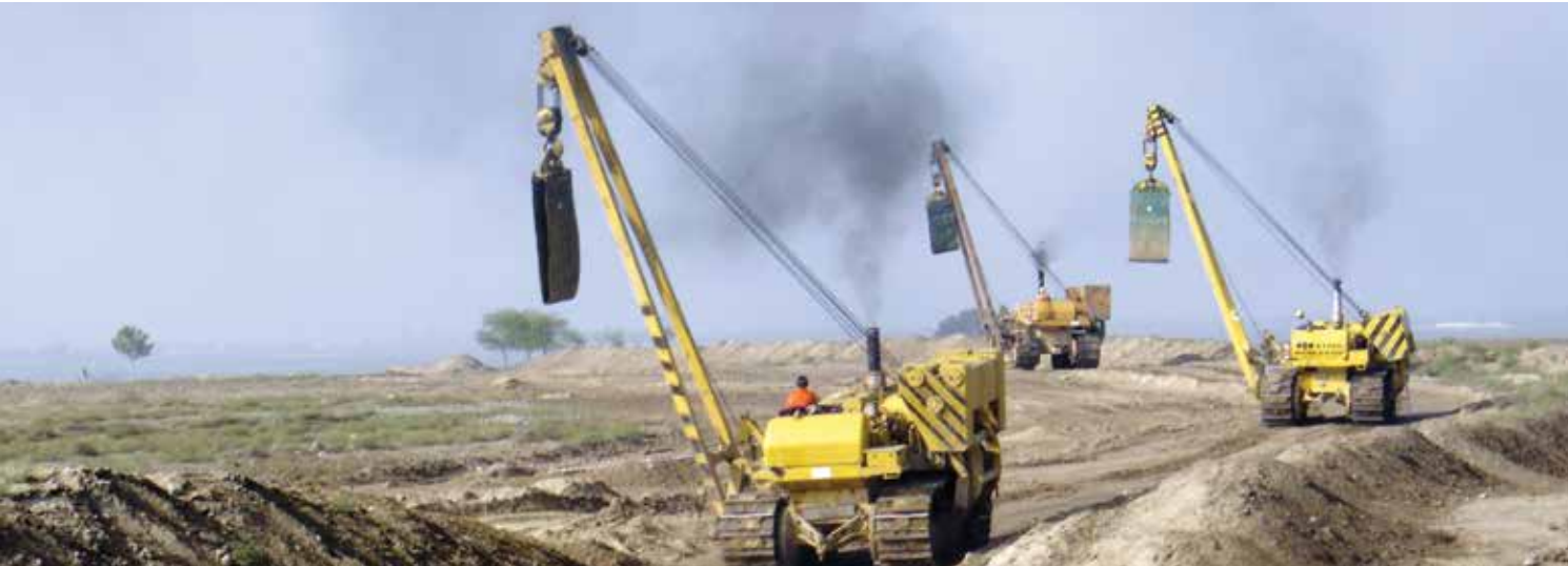
In western Azerbaijan, a group of side booms travel along the pipeline corridor.
